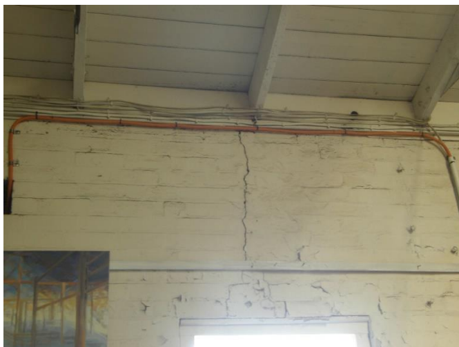
Figure 25 - Detail of typical crack in brickwork in the northern section of the former Pilchers Baking Company building. (NBRsArchitecture, August, 2016)
